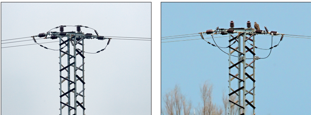
Figure 14. Dangerous jumper in upper position on a 22 kV tower (left) and change of its placement under the plane of main wires (right). Photo: J. Chavko
